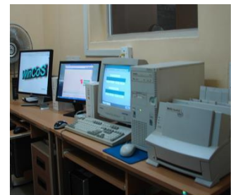
Mill Control Room
